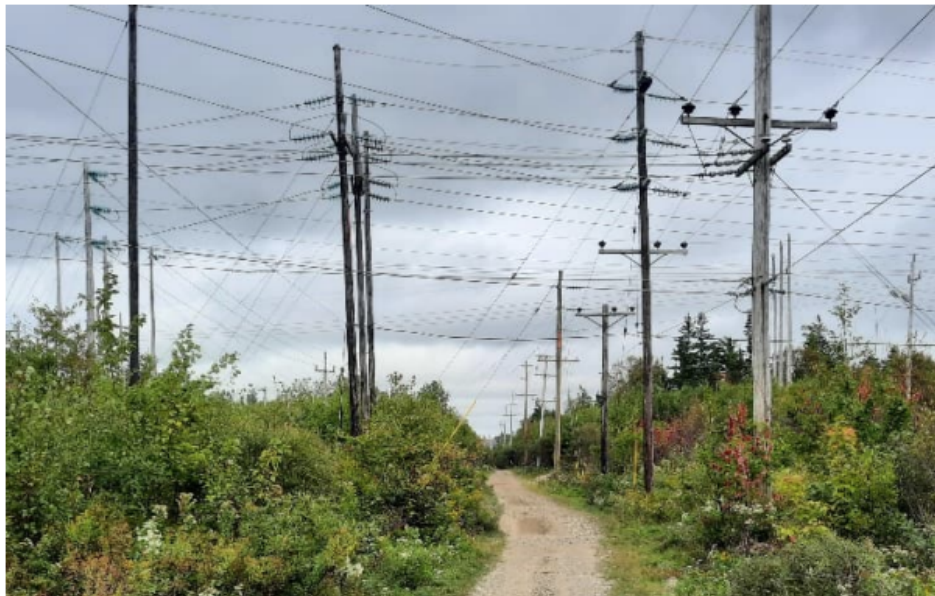
Overhead wires at Old Tramway near CBU.
